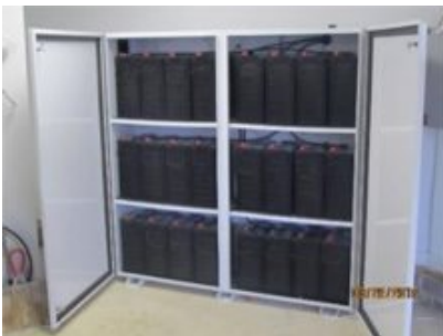
Batteries and Enclosure
