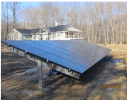
Solar Modules and Racking
