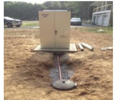
Hydrogen Tank Connected
