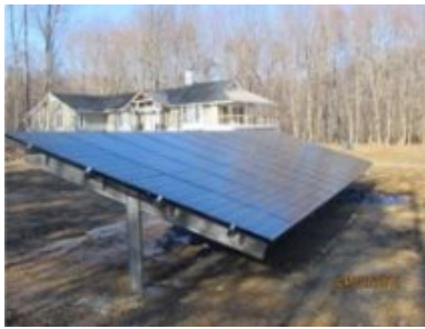
Solar Modules and Racking
