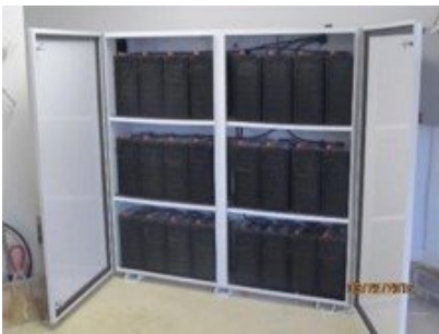
Batteries and Enclosure
