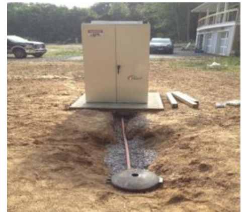
Hydrogen Tank Connected
