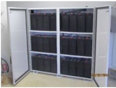
Batteries and Enclosure
