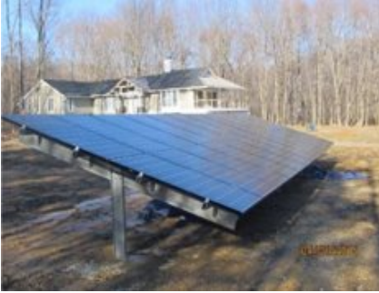
Solar Modules and Racking
